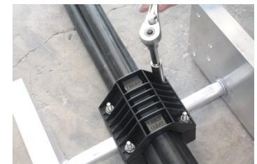
Figure 3 Cable Cleat on Cables and Rung
